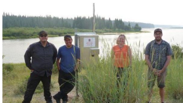
Photo 7: Water monitoring station at Chilcotin Lake for TNG's Water Quality and Quantity monitoring program; station installations were completed in July!
