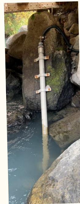
Water monitoring station component: Pressure transducer/temperature sensor in an aluminium pipe
