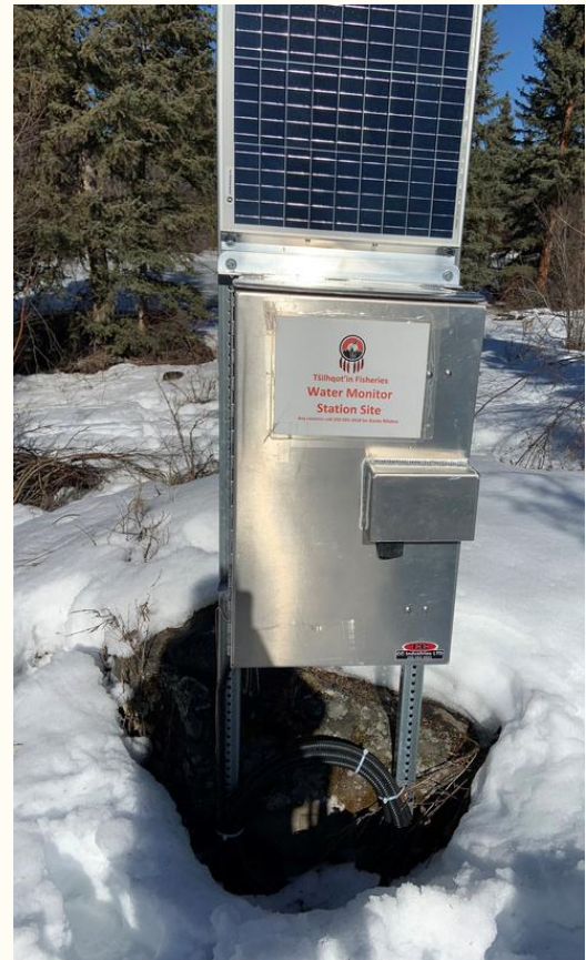
Water monitoring station component: Enclosure with solar panel and antenna.
